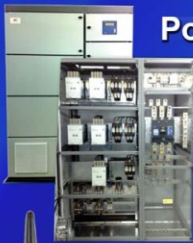
MH Fast Switching Bank
